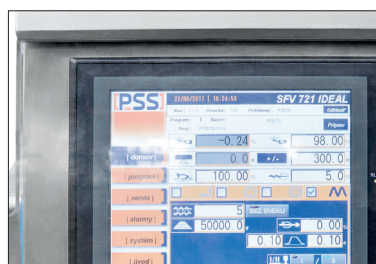
Panel de control central
