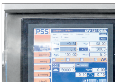
Central control panel
